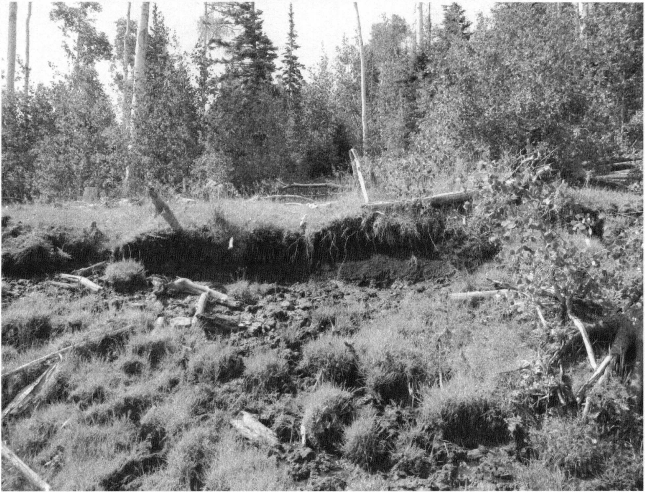
Photograph 9: Water seep and erosion. Photopoint: H UTM Coordinates: 498322 4397504 Bearing of Shot: 169 degrees
