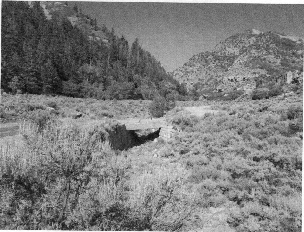
Photograph 37: Bridge on the county road on the Property boundary. This image was recorded after Carbon County bladed the road, which the County claims as a B road, to a width greater than existed at the time of signing the CE.
