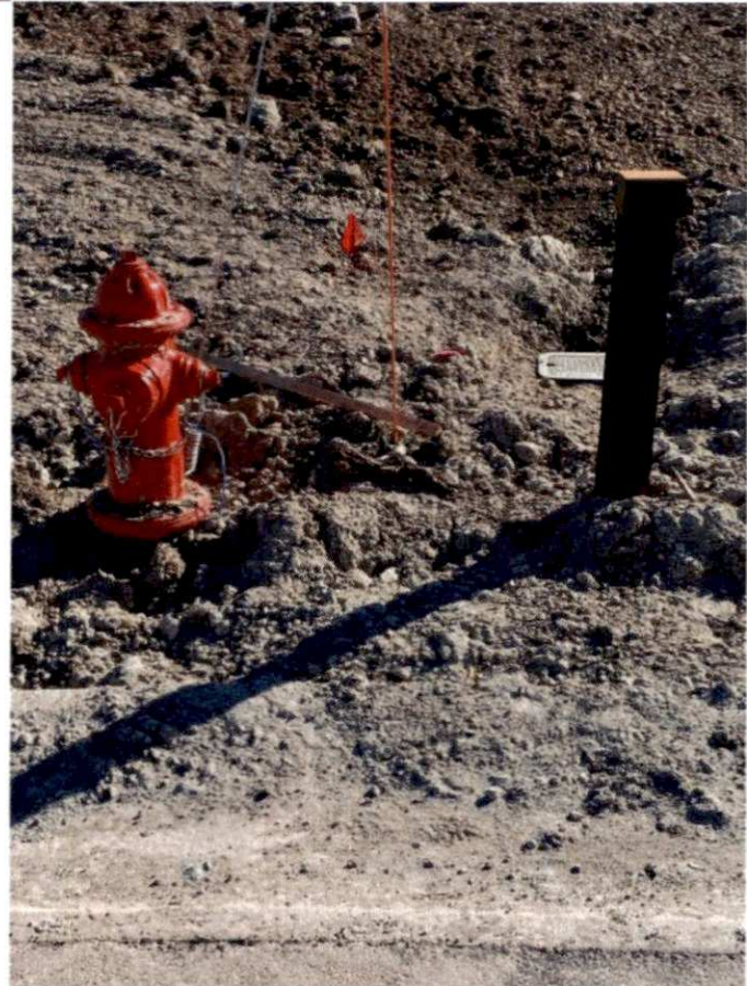
PHOTO EXAMPLE OF CONSTRUCTED FIRE HYDRANT LIGHT BOLLARD
